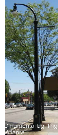
Existing Roadway and Pedestrian Lighting, Fairburn
