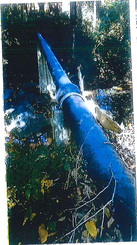
8" uncased pipe crossing stream
