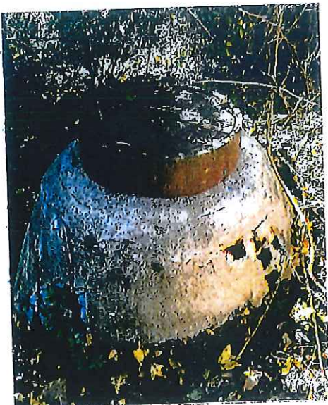
Dilapidated brick manhole
